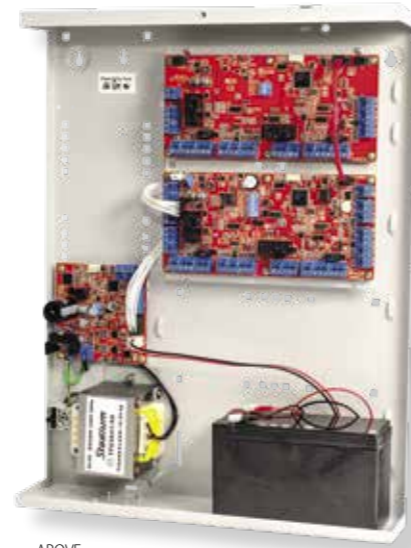
ABOVE: ILAM shown in 4 Door / 4 Reader configuration. (ILAM with UniBus 2 Door / 2 Reader expansion device connected) Housed in the Medium size INTG-995201PEEU3 enclosure with 3Amp SMART Power Supply.
